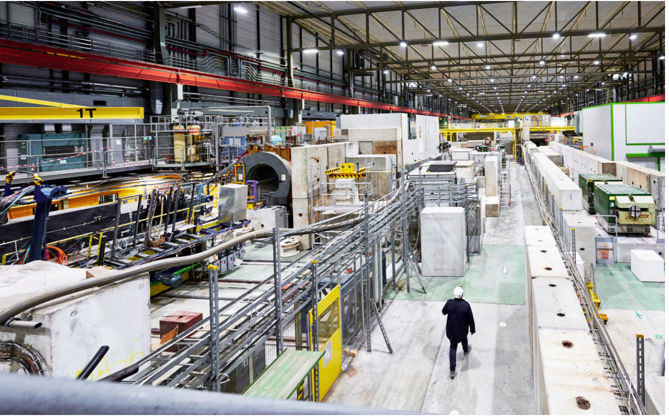
North Area gas infrastructure consolidation
