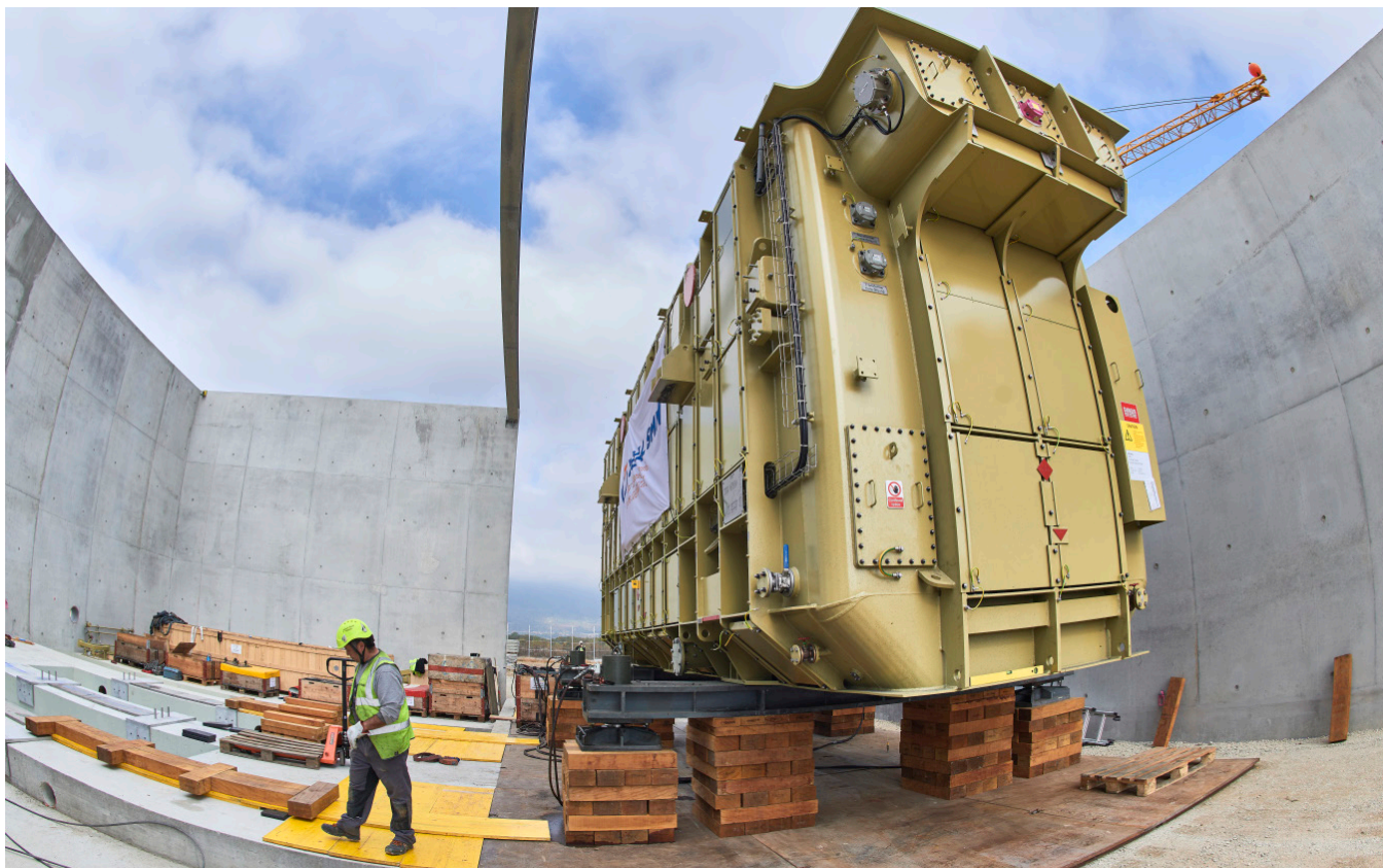
A power transformer in the BE2 electrical substation.
