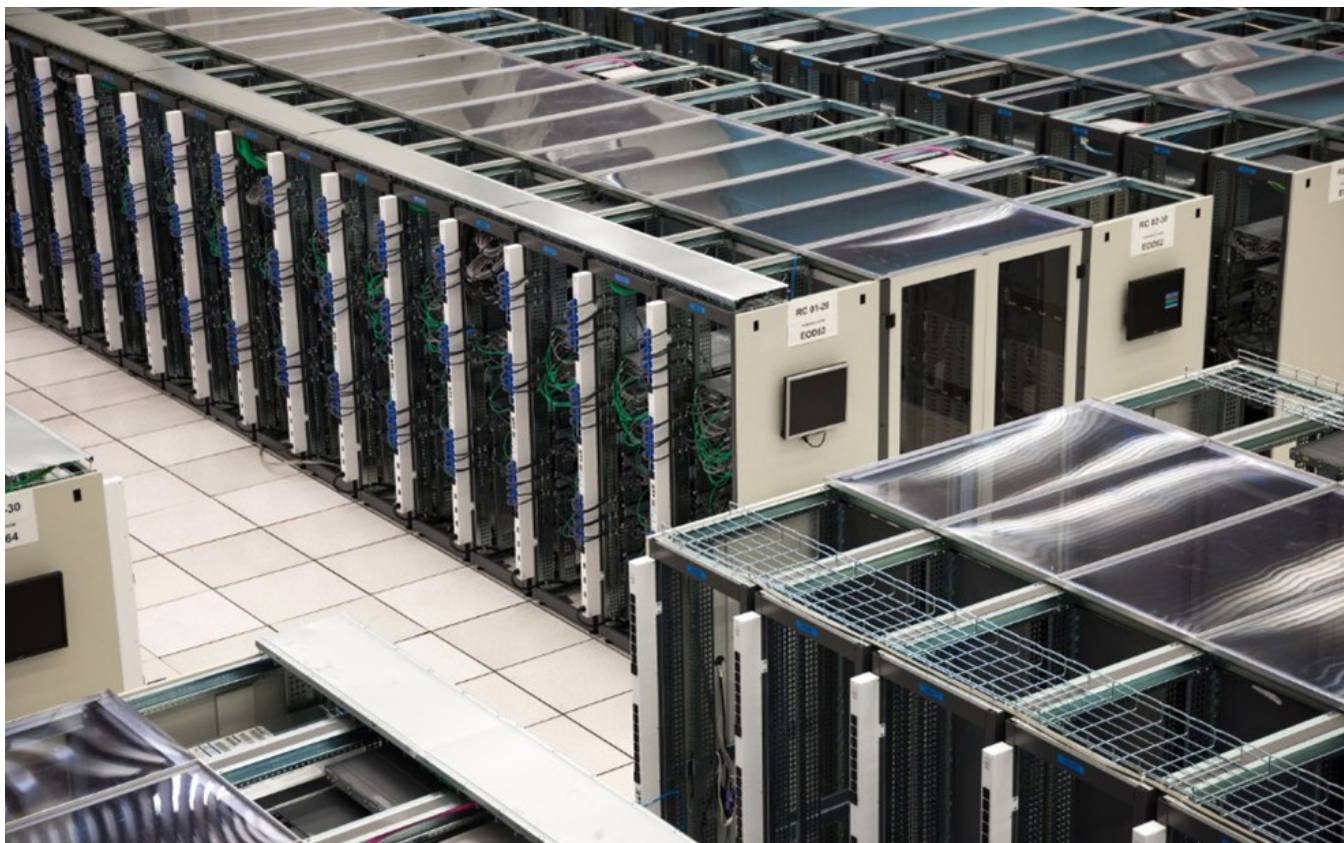
CERN's Data Centre
